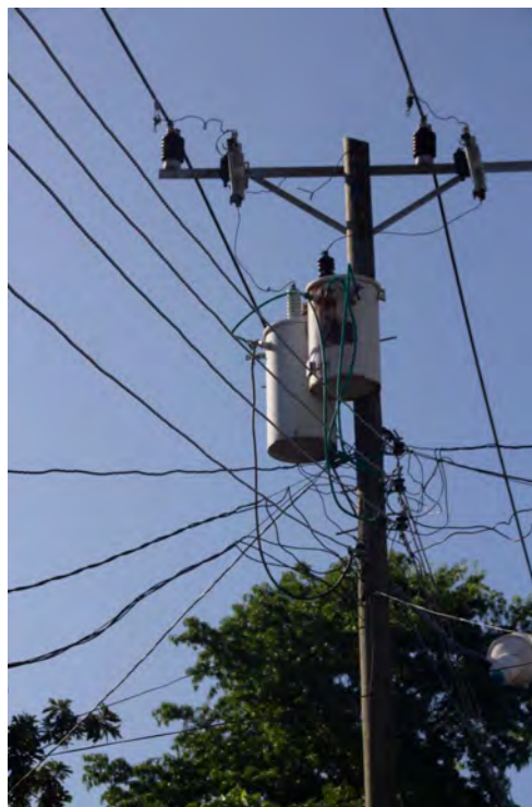
Distribution network transformer
