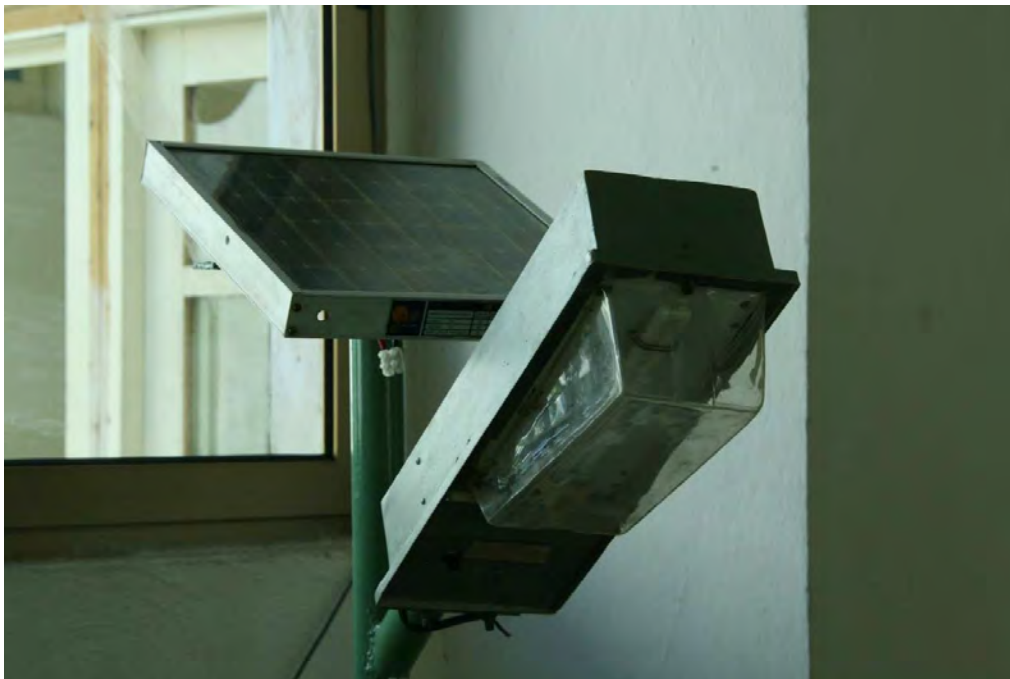
Street lighting with a photovoltaic panel
