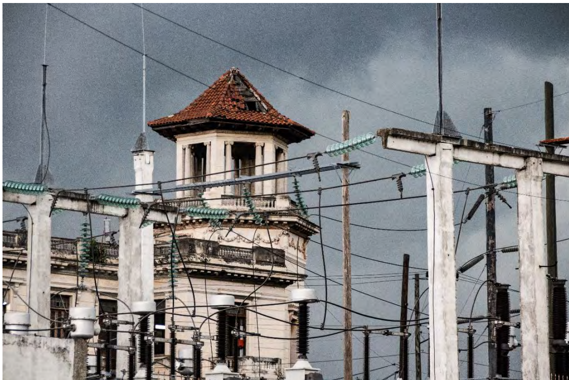
Electricity sub-station, Havana
