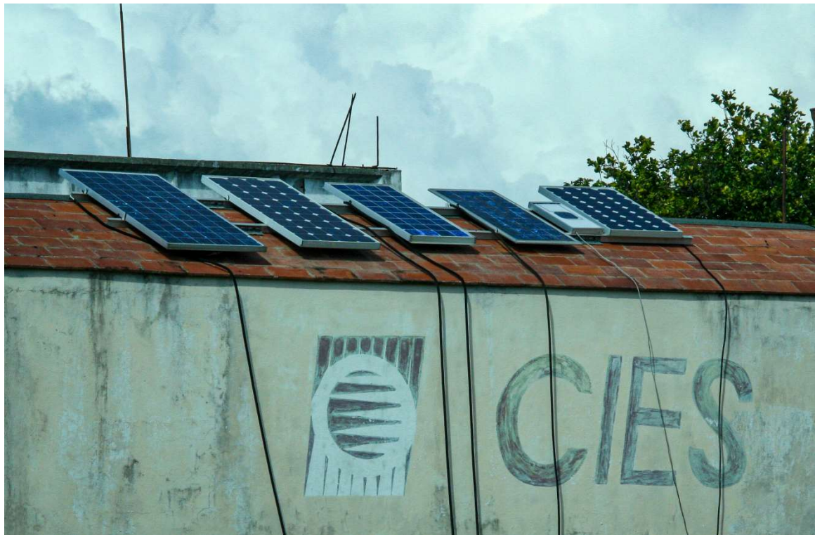
Solar panels, Solar Energy Reseach Centre
