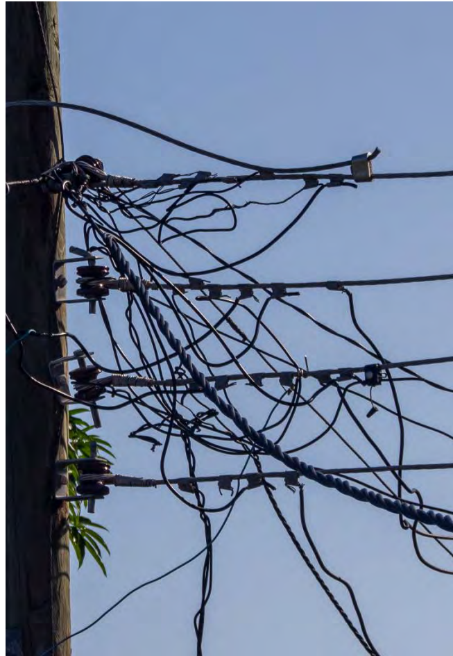
Distribution network installations, Havana
