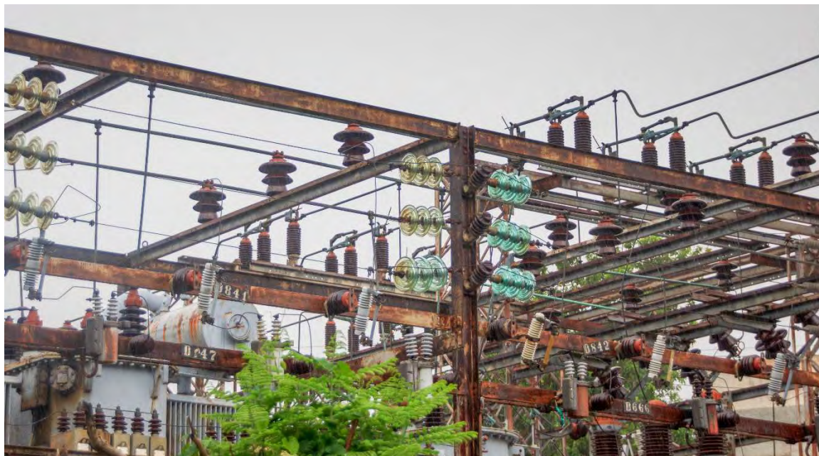
Electricity network sub-station, Havana
