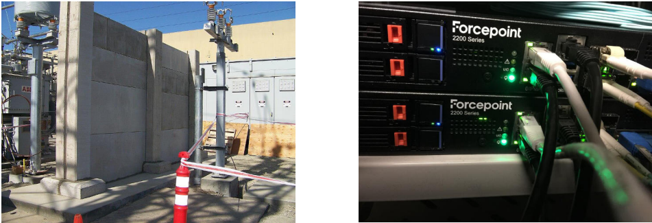
Figure 4. On the left: Electrical Substation Firewall installed between substation transformers. (Credit: Jackson Bishop. This image was marked with a CC BY-SA 3.0 license ( https://creativecommons.org/licenses/by-sa/3.0/deed.en )). On the right: A network firewall cluster with cables attached, connecting the device to internal and external networks. (Credit: Kimmo Talvitie.)
