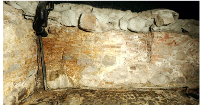
Figure 20. In cellar K94:7, dimension stones were mainly used in the lower parts of the walls. In the photo, you can see the western wall from where four stones were analyzed. All stones are red granite (type 3) quarried from the adjacent Vartiovuori Hill. Photo: Markus Kivistö.
