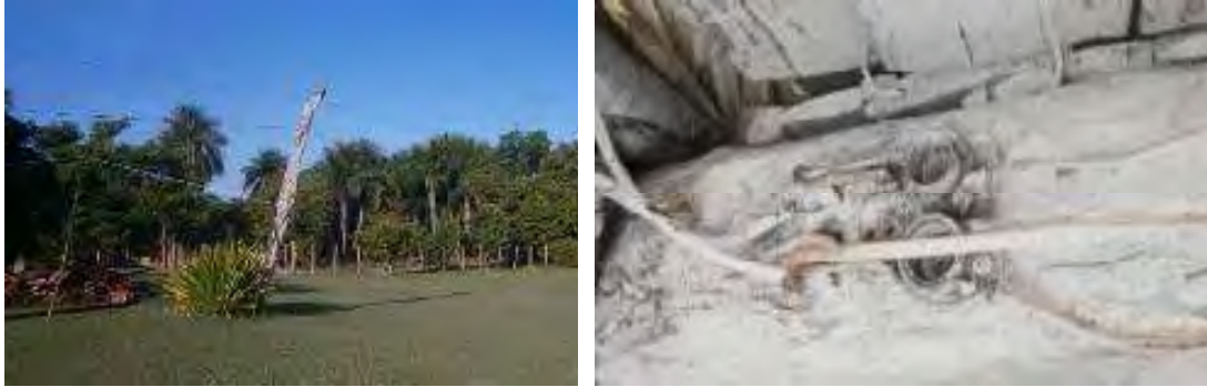
Figure 14. Technical conditions of electric networks in Los Alazanes community. Source: FRE local project.
