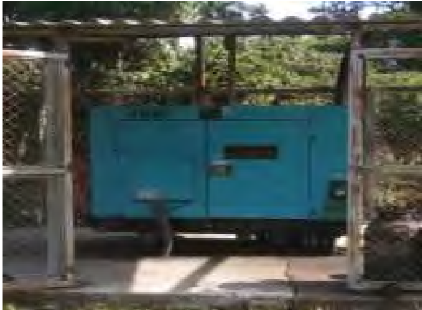
Figure 13. Generator set of Los Alazanes community. Source: FRE local project.
