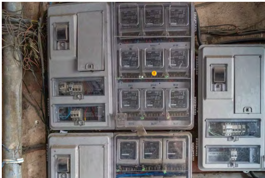
Residential electricity meters, Havana
