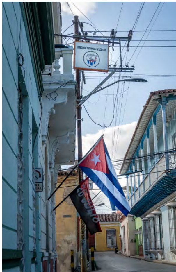
Local electricity distribution, Santiago de Cuba
