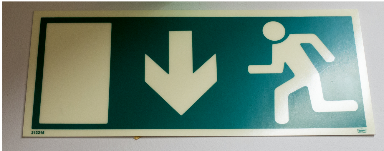
Figure 7. An emergency exit sign mounted on a wall
