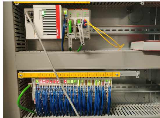
Figure 4.4: Picture of used Beckhoff PLC
