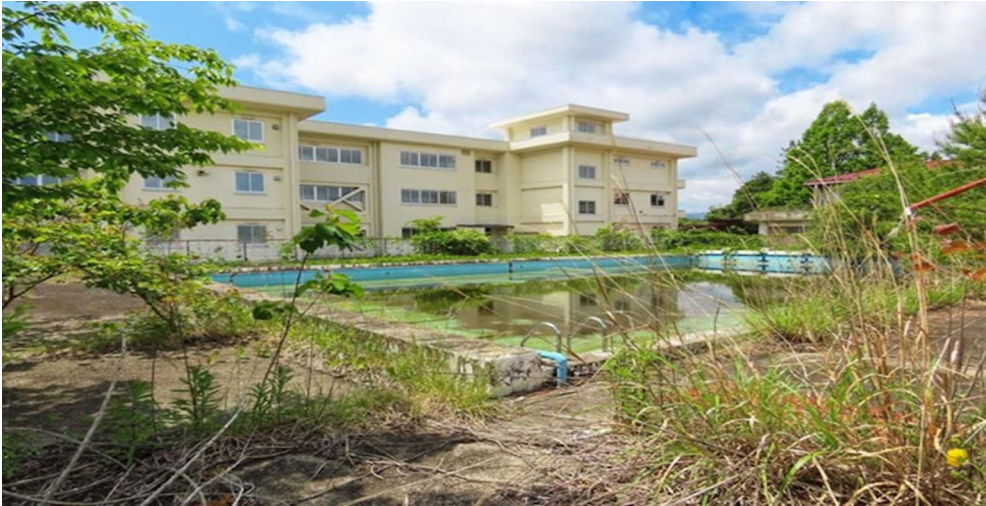
Figure 22. An abandoned elementary school is waiting to be demolished in Namie, Fukushima. Photographed taken in May 2025 by Veera Ojala.
