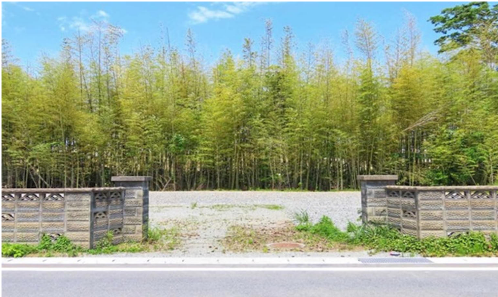
Figure 13. A site in Okuma town where the former housing infrastructure is demolished. It can be classified as “Zones Being Prepared for Lifting of Evacuation Orders” as the decontamination and demolition work is finished. What will be here in the future is open. Photographed in May 2025 by Veera Ojala.
