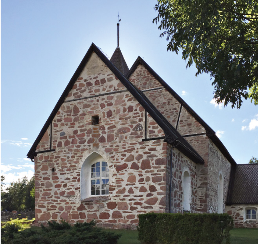
FIGURE 7 Hammarland church with both tie beam truss and rafter foot truss visible in the gables
