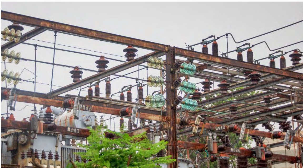
Electricity network sub-station, Havana
