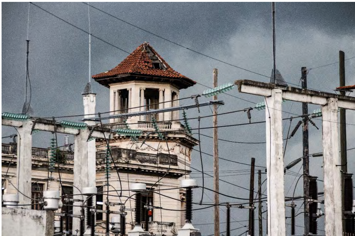
Electricity sub-station, Havana
