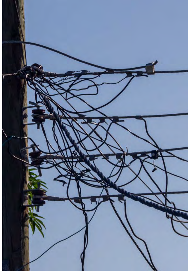
Distribution network installations, Havana
