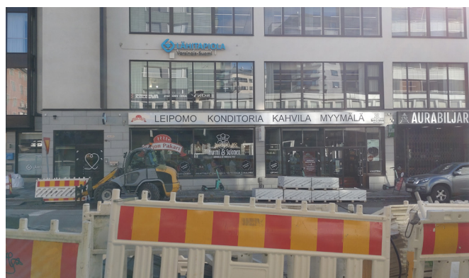
Fig. 10. A recently established bakery & café in August 2022 in the middle of the construction work [photo by the authors].
