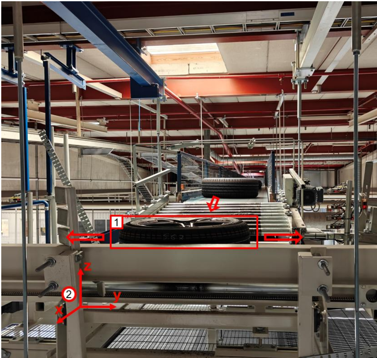
Figure 15. The tire separation point on the tire conveyor, where the machine vision system could be implemented. Box 1 represents the location where tires stop before being separated to their respective conveyors, and circle 2 indicates the axis along which system specification data is defined. From: the author (2026)
