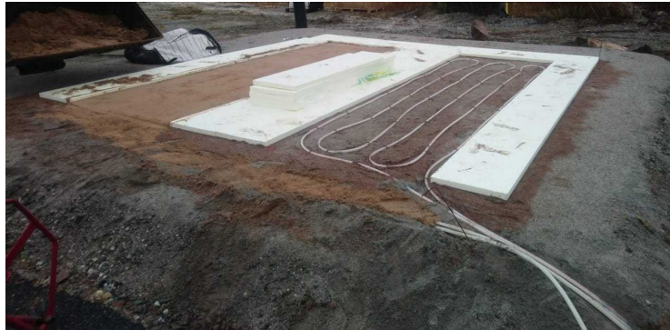
Figure 4: Inner pipe arrangement of the active cooling system of Group B .
