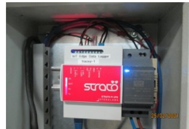
A picture from the main engine where the StratoPI is connected to the NORIS data gateway, and the vessel's LAN.
