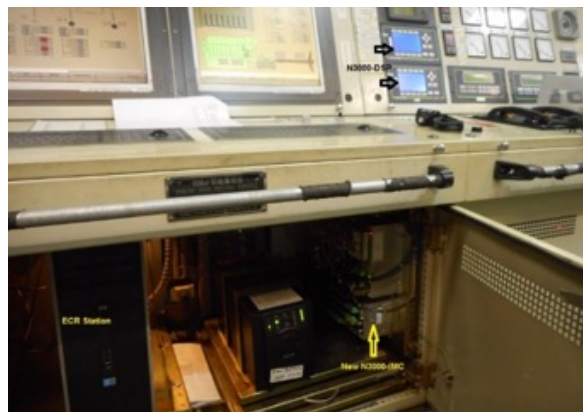
A view of the NORIS 3000 alarm system in the engine control room on one of the Lauritzen vessels.
