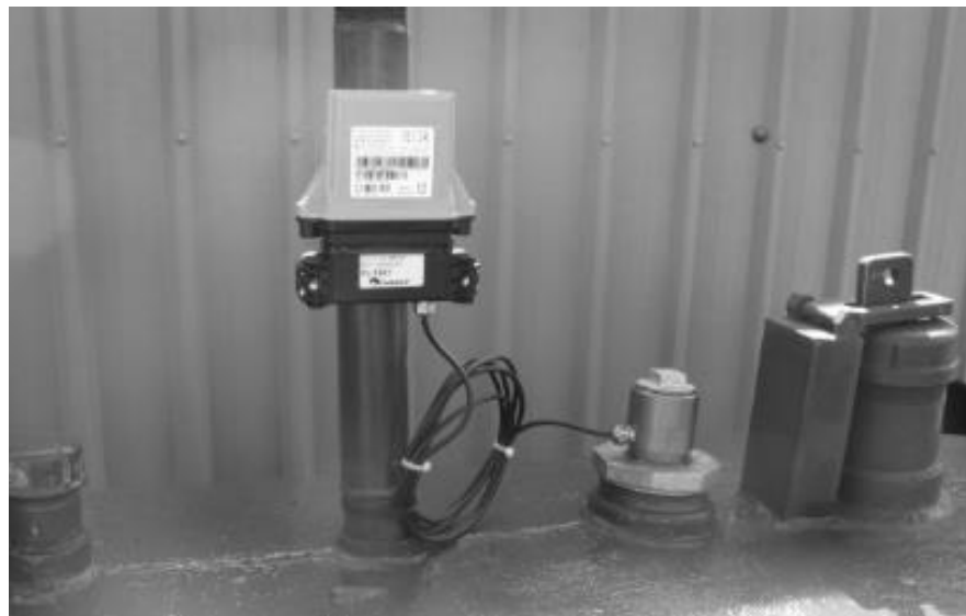
Figure 4- Sensile's oil and lubricant tank-level telemetry system (Direct quote from [20]).
