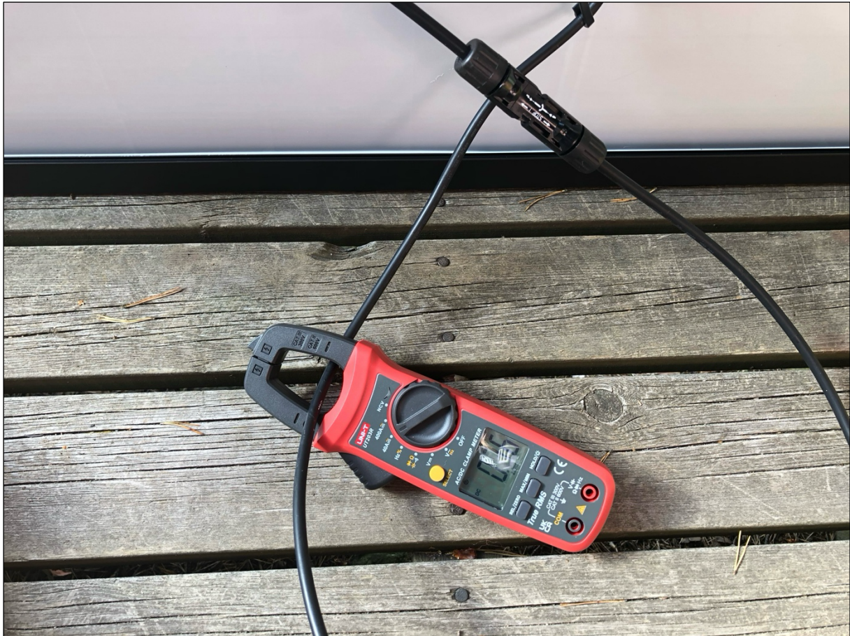
Picture 48. Measurement of closed-circuit DC using a clamp meter (Viljami Kukkola)
