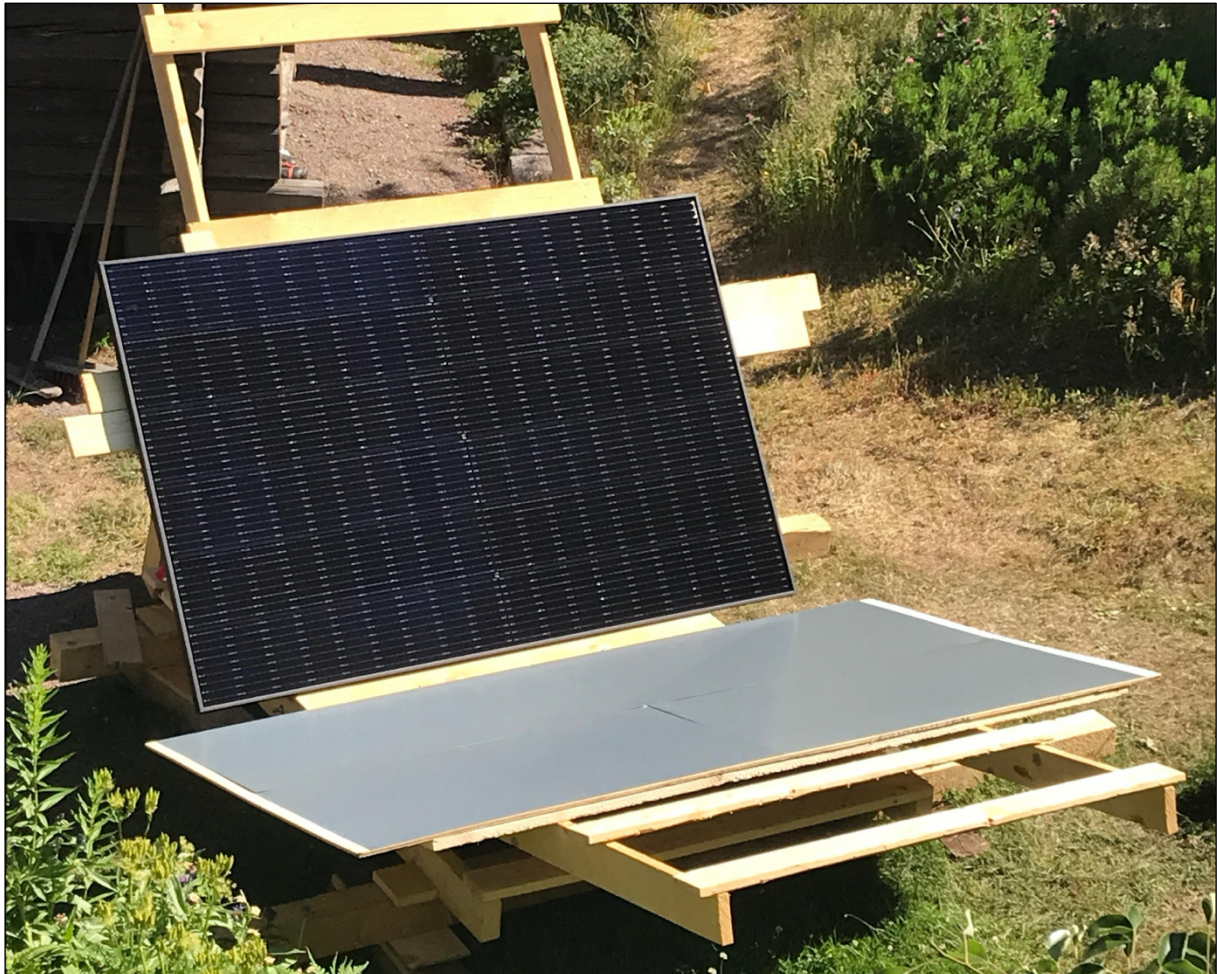
Picture 46. Solar panel and reflector of the experimental setup. (Viljami Kukkola)
