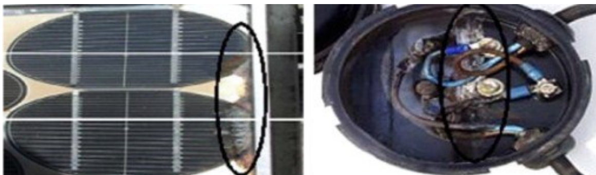
Figure 5. Solar cell corrosion (left) and corroded cables inside junction box (right) [2]
