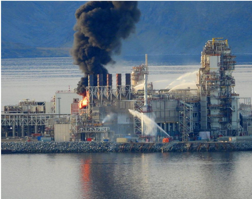
Figure 3.4 The turbine on fire at the Hammerfest LNG plant in September 2020
